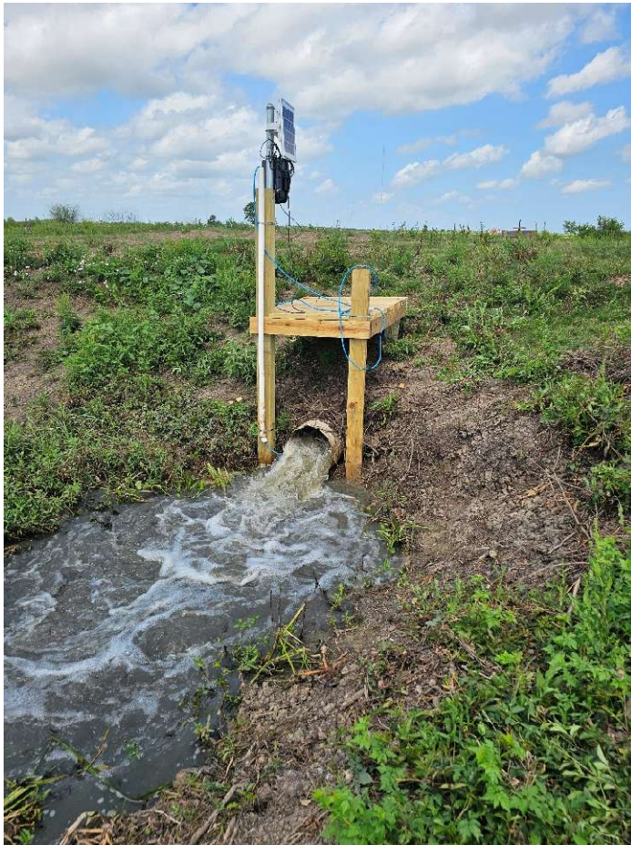
Figure 3. Diversion point with water meter measuring water velocity, flow rate, and water volumes diverted from irrigation canal.
